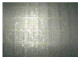
SCR Exit—Catalyst Entrance Inspection
