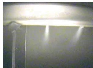
SCR Exit—SBS Injectors Inspection
